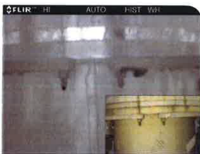
Visible vs. OGI image of SF 6 leak
