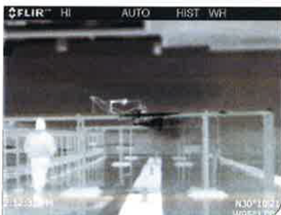
Ammonia (NH 3 ) gas escaping from pipes
