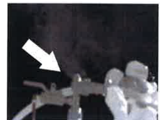
Captured SF 6 leak
