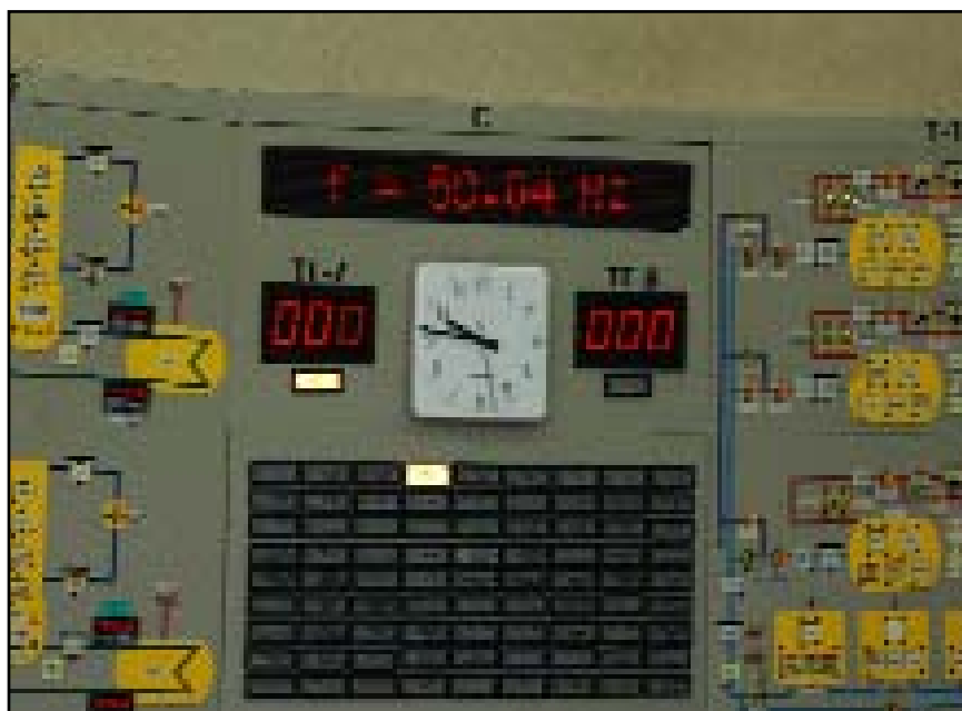
Indicators show zero power of turbine generators 7 and 8
